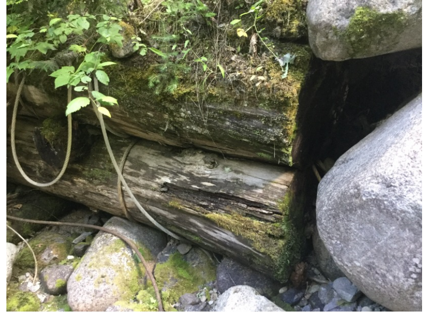
Left Abutment Downstream Corner Fungal Growth
