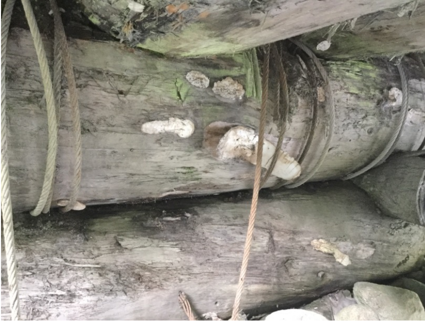
Right Abutment Crib Fungal Growth
